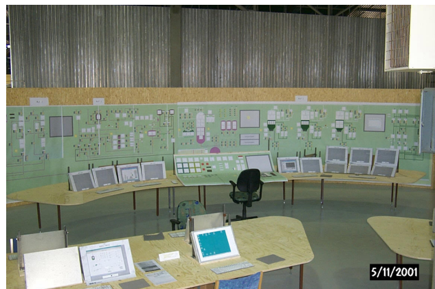
Figure 2 - A Wide Angle View of the Control Room
